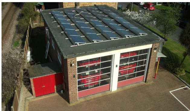
Figure 12 – Solar panels at Frinton Fire Station.
